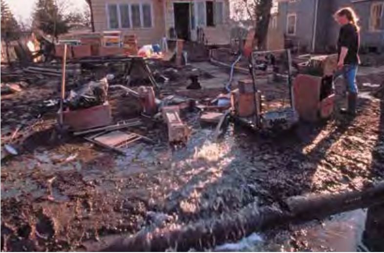
Cleaning up after a basement flood Photo Courtesy of Michael Reiger
